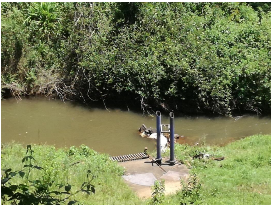
Plate 9. Intake chamber at River Kimakia
