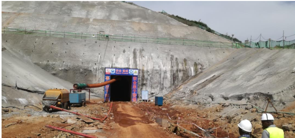
(i) concrete facing for the outlet of the tunnel at Karimenu II Dam
